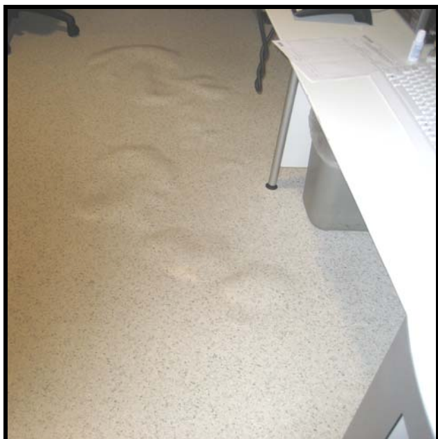
Blistering in Non-Permeable Vinyl on a Wet Slab
